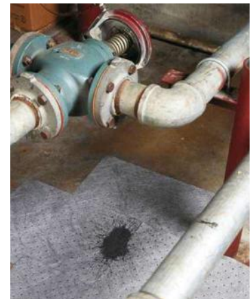
Use pro-actively to catch leaks and drips.
