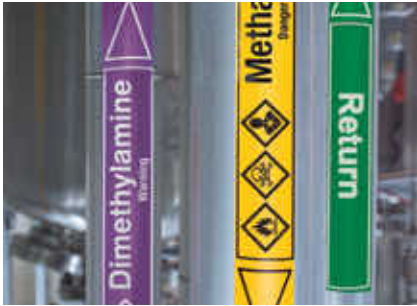
Pipe & valve marking
