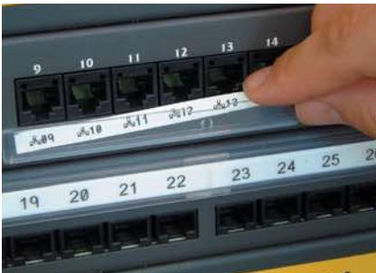
Punch block & patch panel labels
