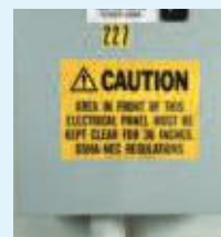
Hazard warning signs
