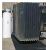
Ideal underneath leaking transformers.
