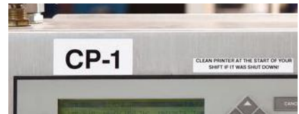
Control panel & electrical panel labels
