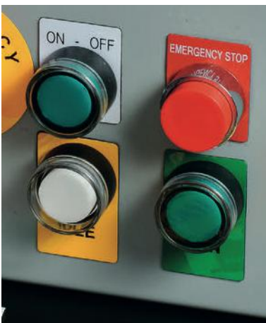
Control panel labels
