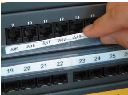
Punch block & patch panel labels
