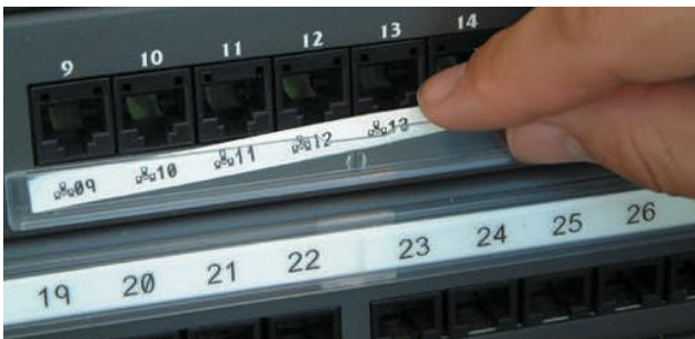
Punch block & patch panel labels
