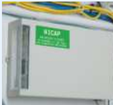
Control panel labelling
