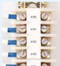
Terminal block marking
