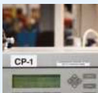
Control panel and electrical panel labels
