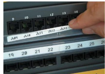
Punch block & patch panel labels
