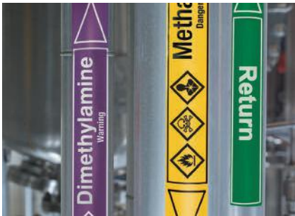
Pipe & valve marking
