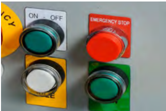
Control panel labels
