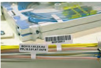
Fibre optic cable markers
