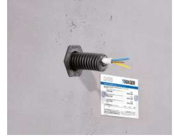
Wall feed-through in concrete fire-protection wall.
