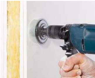
Cut an installation opening using a Ø 74 mm cutter (e.g. MULTI 4000: Art. No. 1084-10).
