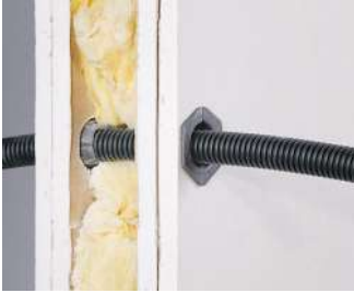
Wall feed-through in plaster-board fire-protection wall.
