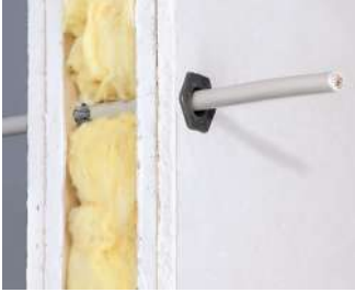
Wall feed-through in plaster-board fire-protection wall.
