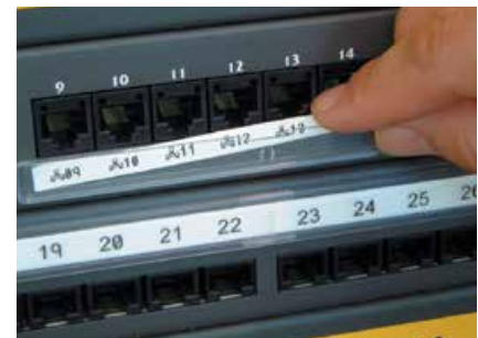
Punch block & patch panel labels
