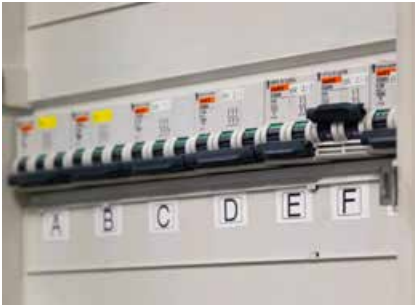
Circuit breaker marking
